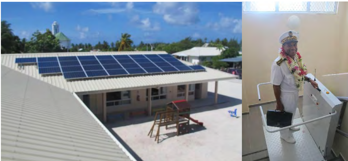
Installation photo voltaïque
